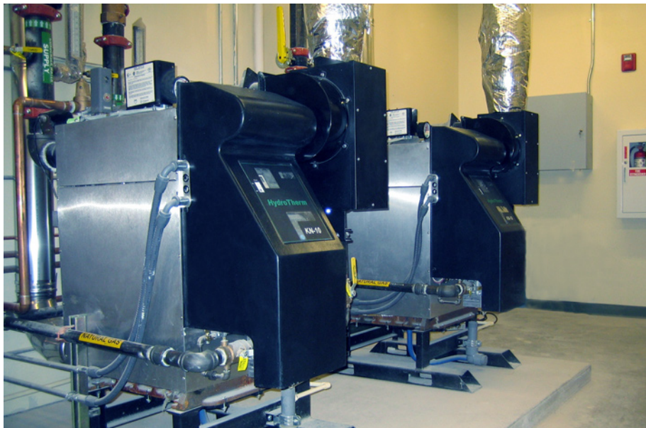
KN-10 condensing boilers were ideal for the low temperature hydronic system at Hunter Elementary School
